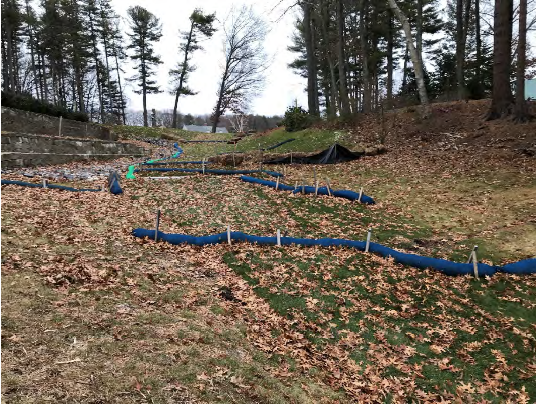
Fig 11: Slope below the manhole at Gundalow Landing/east side of the bay. Viewing east. (01-11-21)
