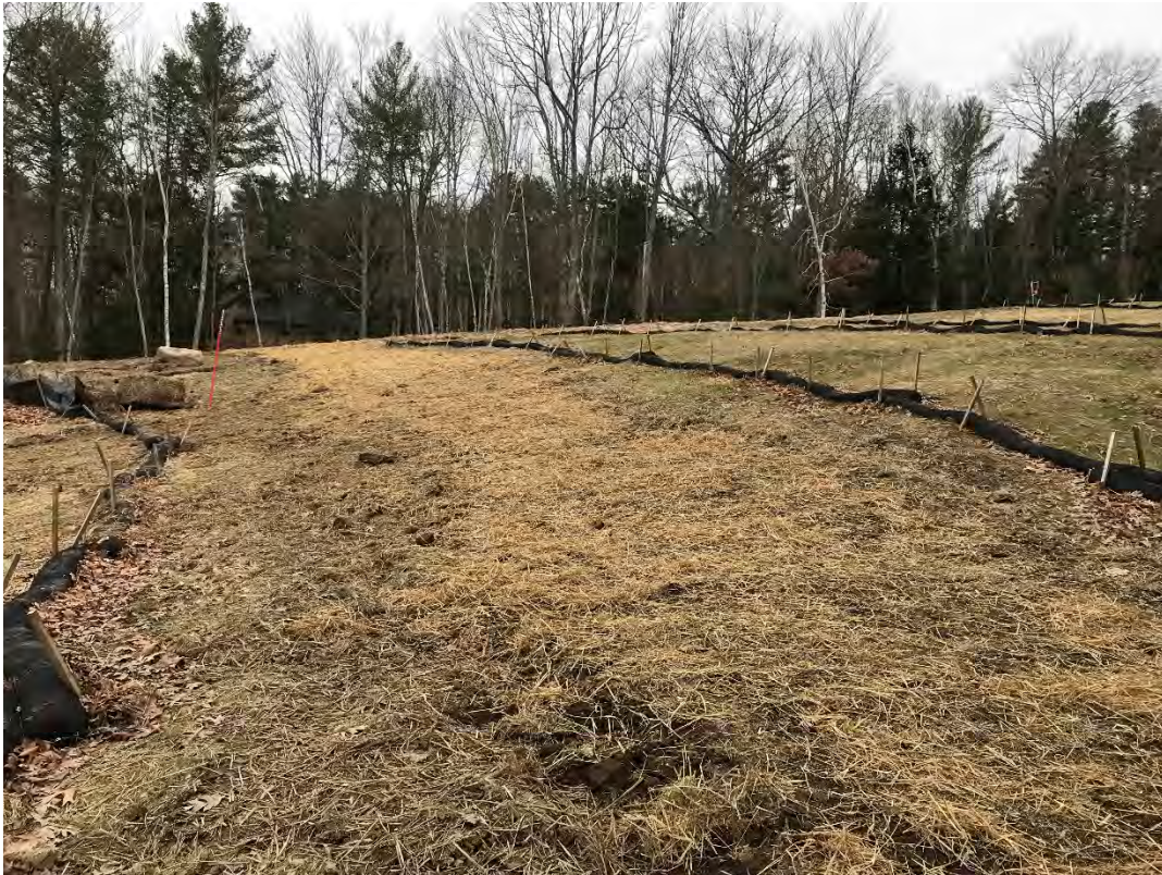
Fig 1: Stabilized access across the slope above the cable house at the Eversource property/west side of the bay. Viewing southwest. (01-11-21)
